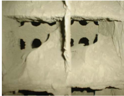
Ammonium bisulfate on preheater
